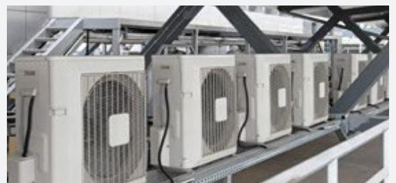
Outdoor Equipment of air conditioner
